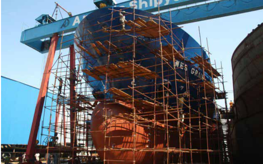
A commercial vessel is being built in Ananda Shipyard and Slipways Limited (ASSL)
